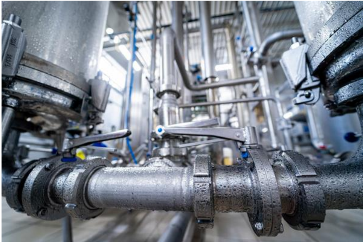
Figure 2: Condensation on a pipe in a brewery © stockfoto
